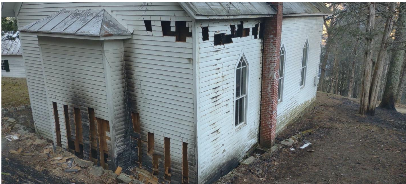
Figure 6. 2024 Fire damage on the outside at Mt. Zion Lutheran.
