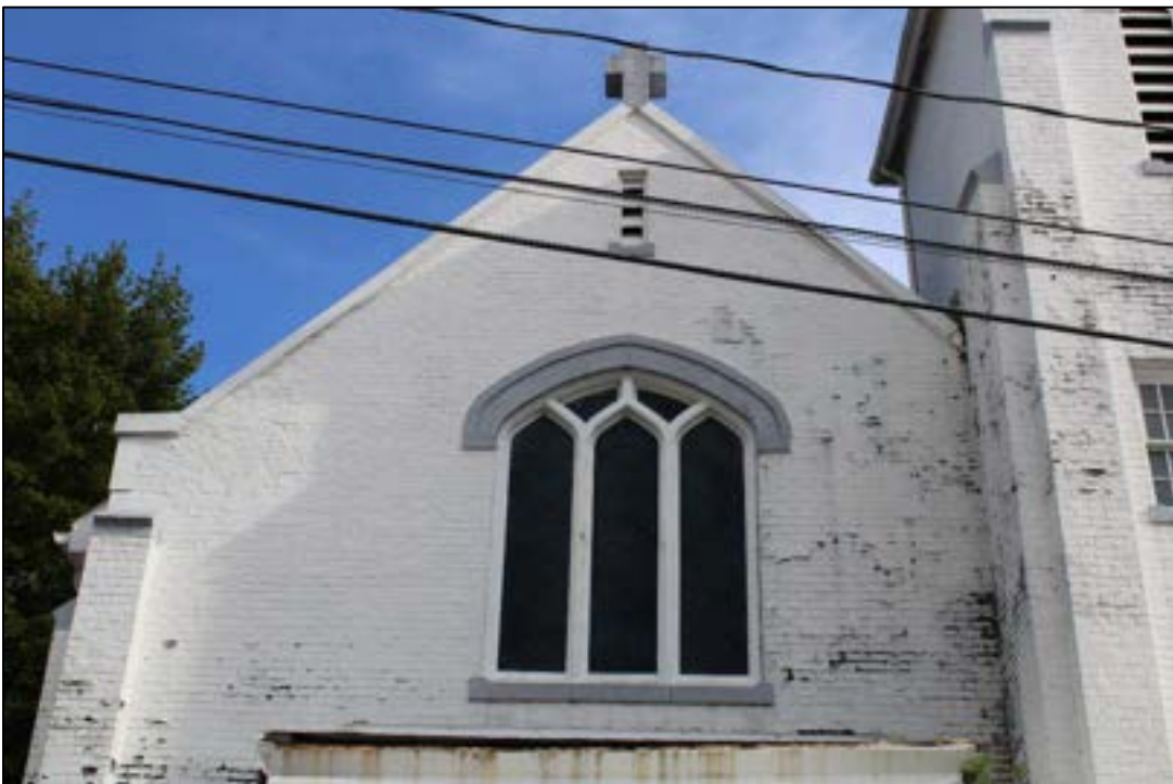
Photograph 4. MC-1215, John Stewart United Methodist Church, 102 Jones Street, Window Detail, Facing Southeast.
