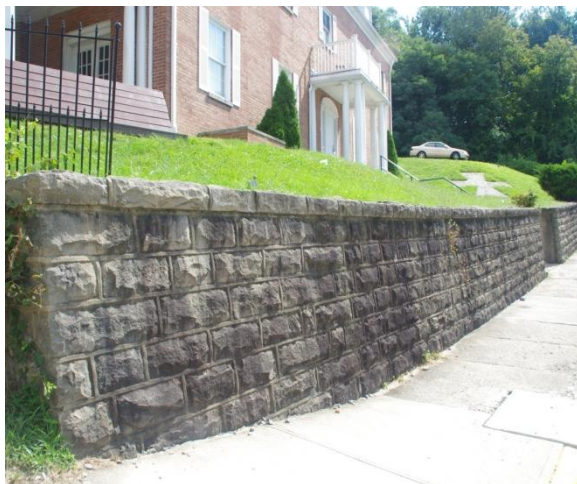
Fig. 12. 700 N High St and Fife Ave MG-2392
