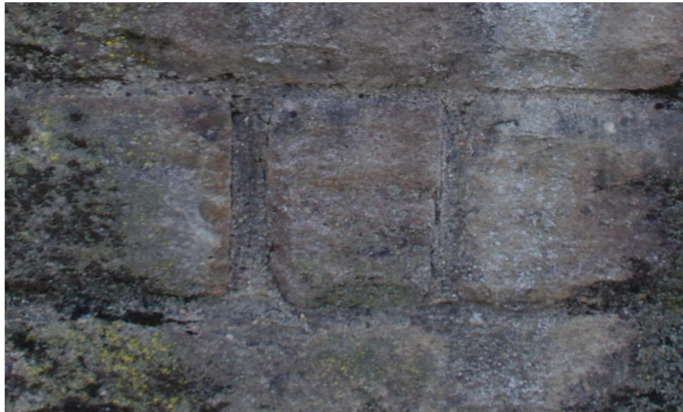
Fig. 4. Joint used in wall at 728 Richwood Avenue located a few blocks from The Richwood Avenue Wall - Vol. II
