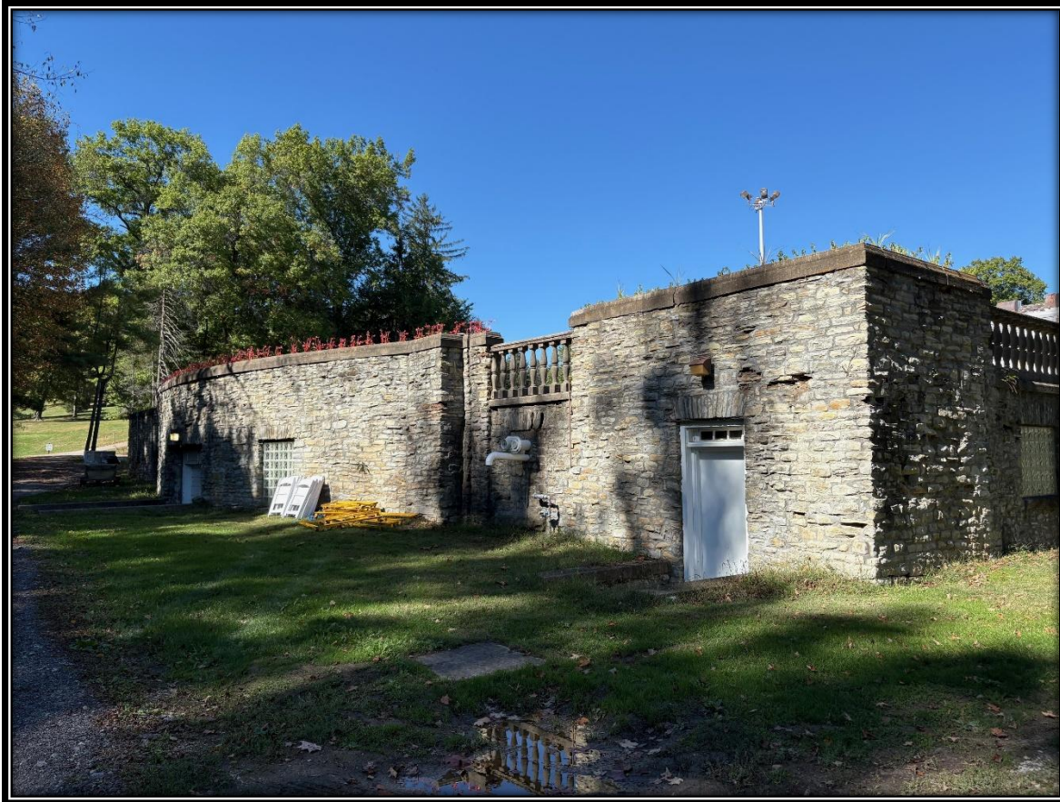
Photograph 28 of 32. The south (rear) and west elevations of the swimming pool foundation, facing northwest.
