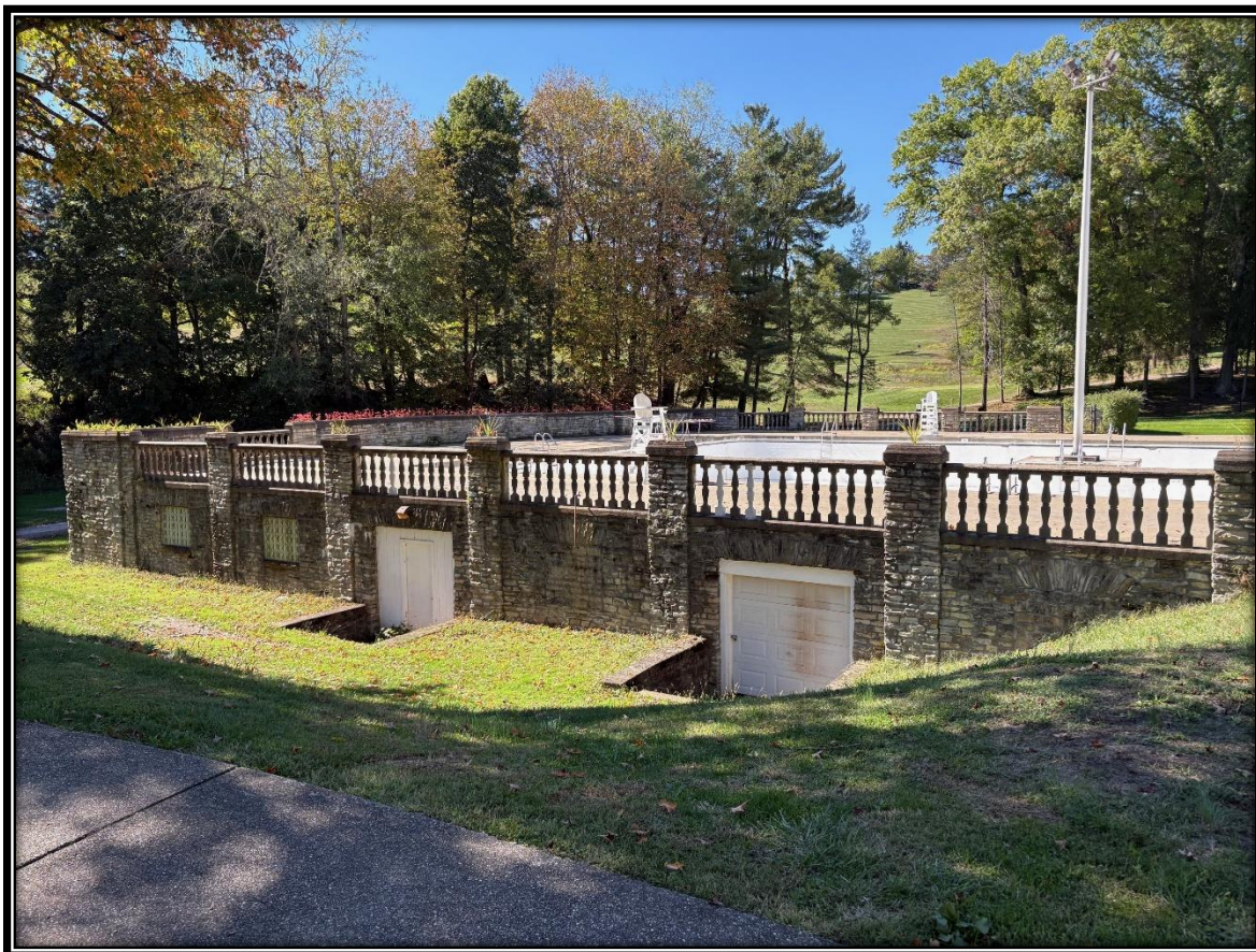
Photograph 27 of 32. The east elevation of the swimming pool and its foundation, facing southwest.
