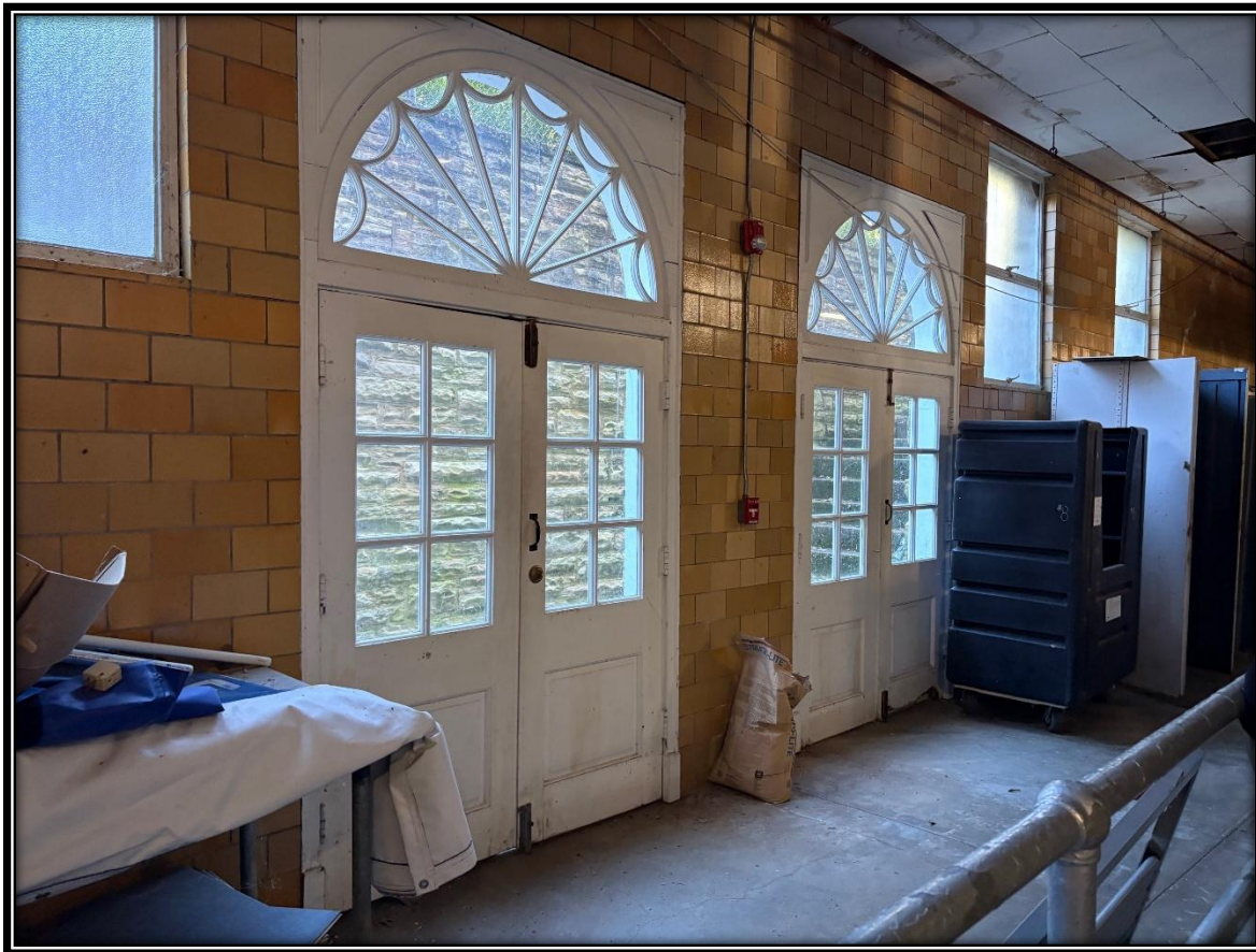
Photograph 4 of 32. Detail of the ground-level entrance doors (from the interior), facing northeast.
