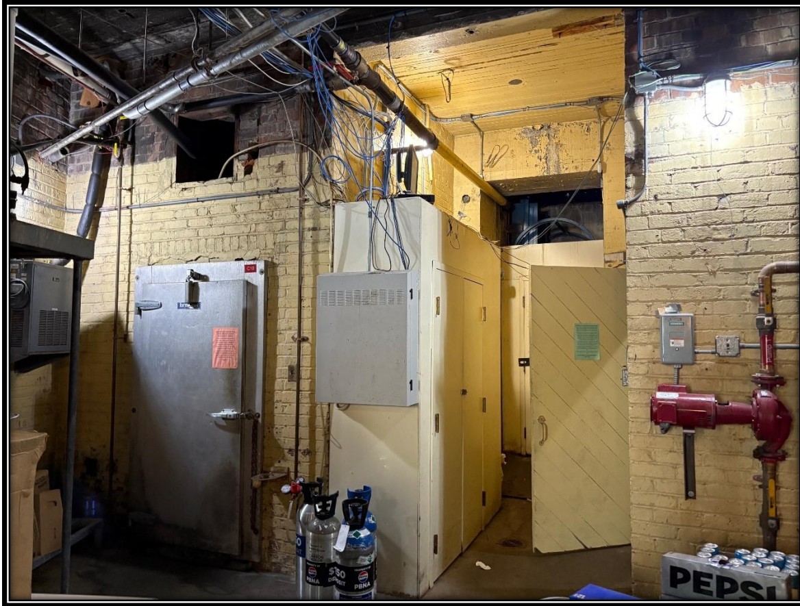
Photograph 18 of 32. The boiler room, facing northwest.
