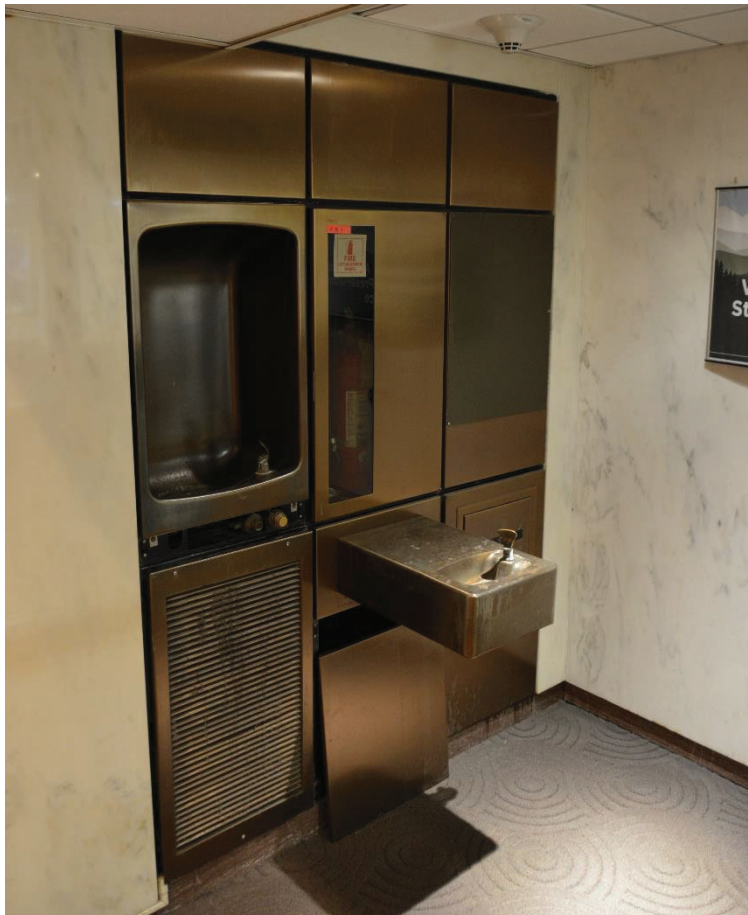
Photo 47 Interior, second story bronze drinking fountain, camera facing southeast
