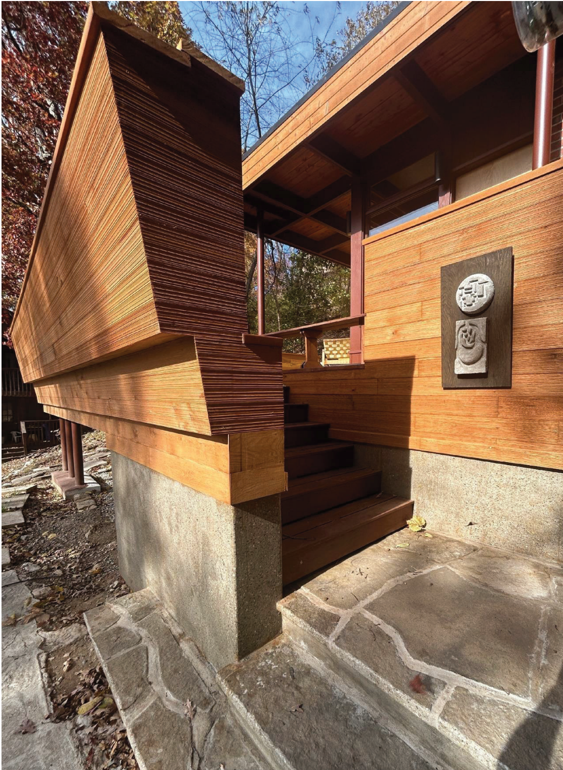
Photo 5 Depicts the ground level stair entry to the deck and details the complimentary deck wall built to match the original cedar siding on 2nd level exterior. Camera facing northwest.
