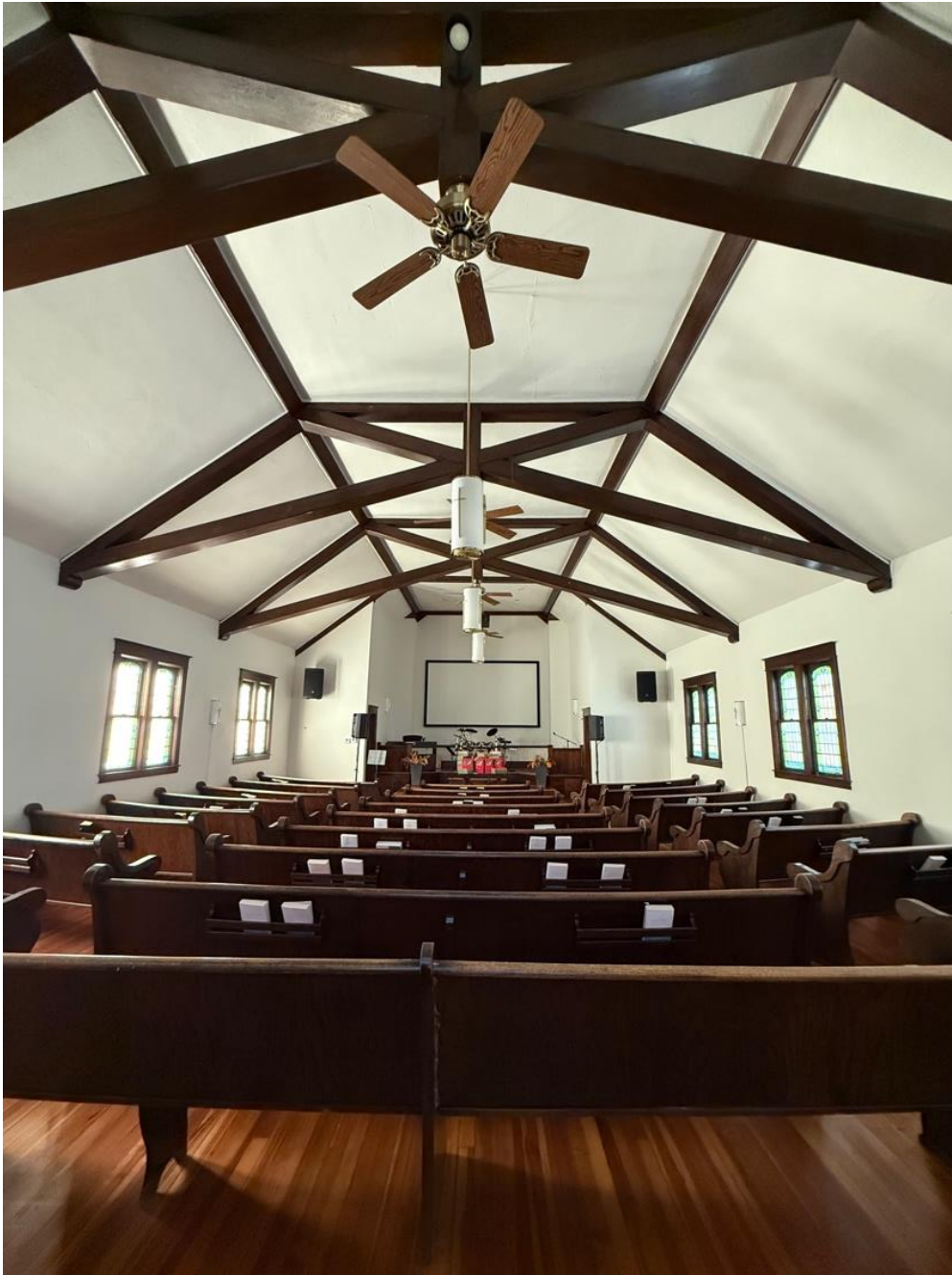
Photo 10: Interior view of sanctuary, facing stage and back of pews; camera facing south.
