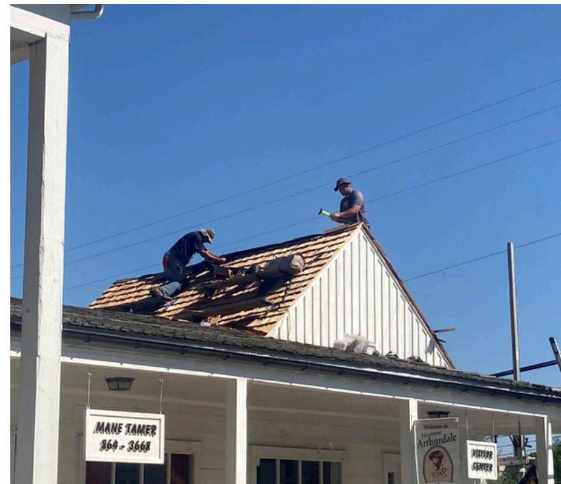
Roof replacement funded by WV SHPO grant in Arthurdale, Photo courtesy of Elizabeth Satterfield, 2023.
