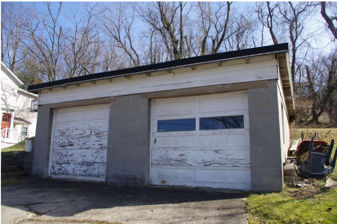
Photo 8: Front view of the two-car garage at 2 Cayton Street, camera facing east.
