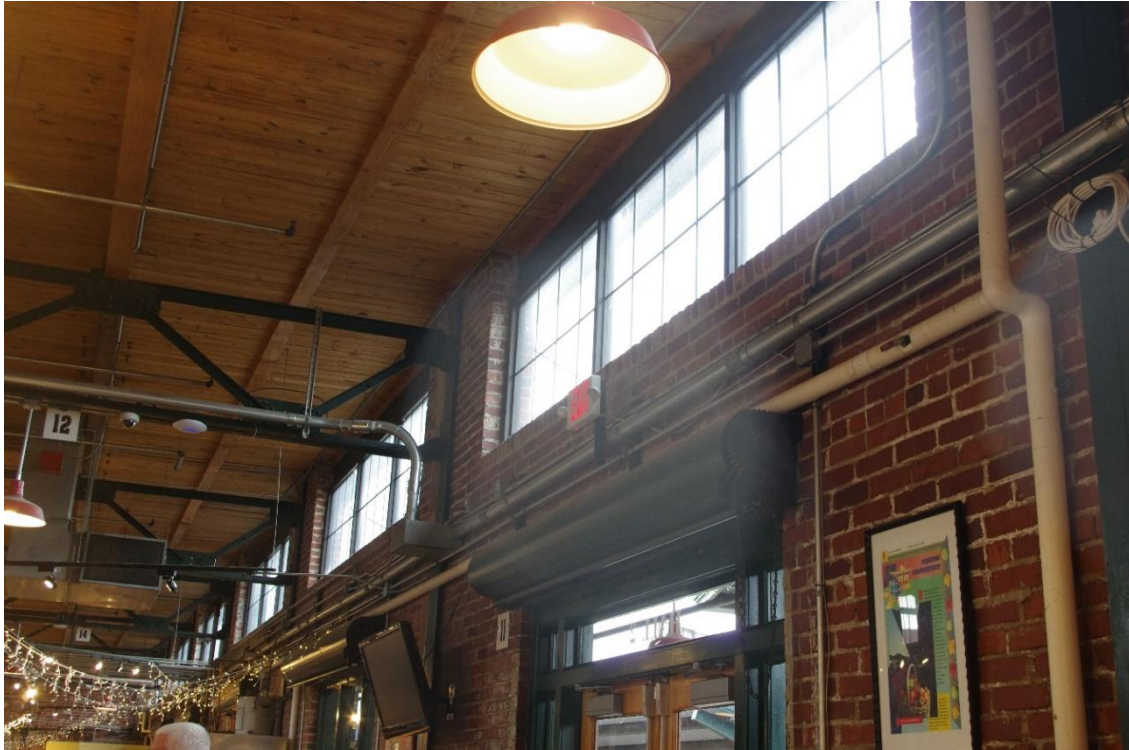
Photo 9. Interior view from center of building showing roof structure and clerestory windows on northeast elevation, camera facing NW.
