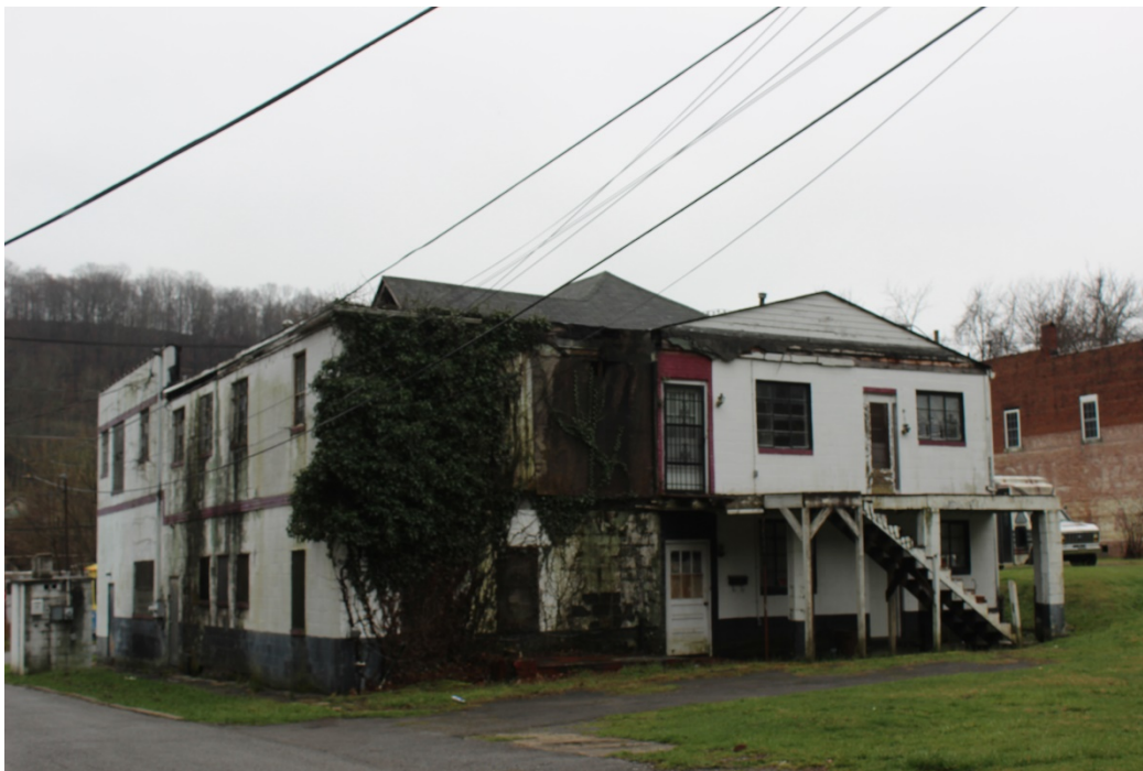
Photo 6: Side (east) and rear (north) view of Hotel Thelma, camera pointing southwest.
