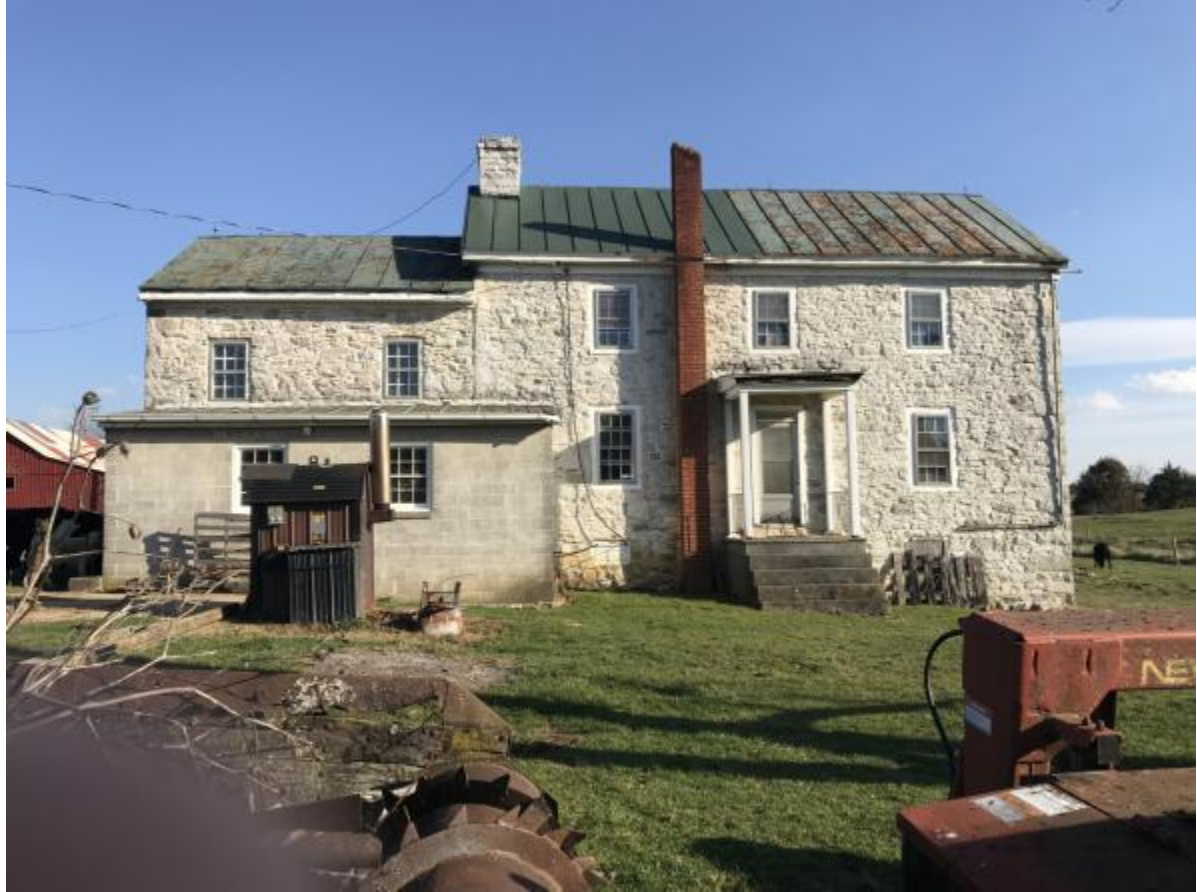
WV_Jefferson County_Rosenberger/Brown Farm_0004. View to south. Unlike five-bays of the front of the main house, the rear has only three, no doubt a cost savings. A modern furnace is attached to the brick chimney. The concrete block addition to the addition houses a modern kitchen.
