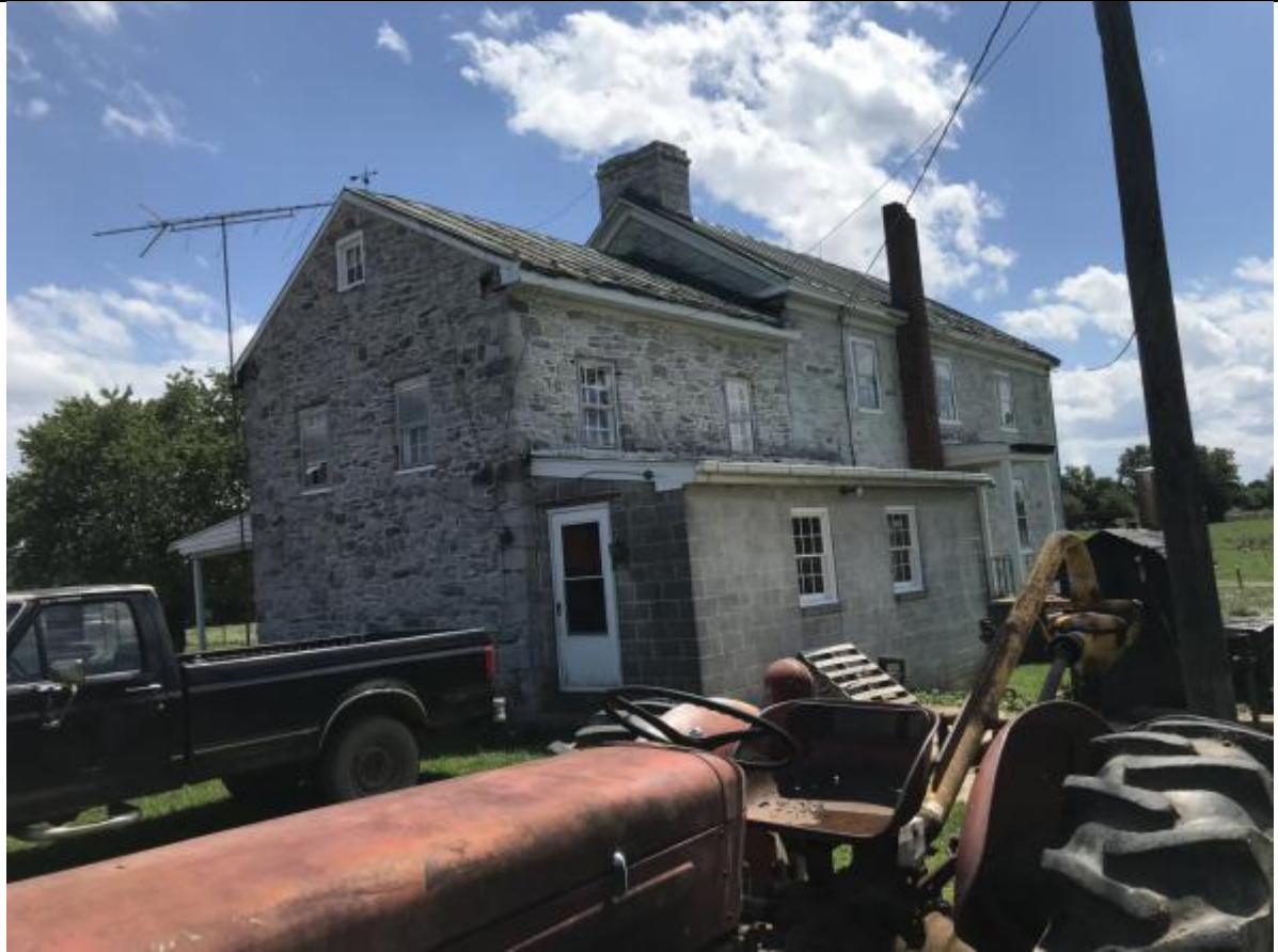
WV_Jefferson County_Rosenberger/Brown Farm_0003. View to southwest. Although the addition has corner blocks dressed as quoins, uncoursed stone in walls varies in color, unlike the stone in the main house.
