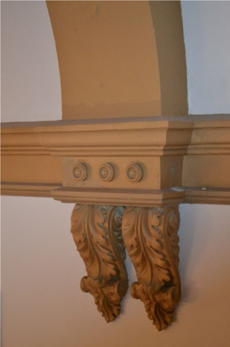
Photo 13. Decorative medallions at the end of the arched brackets. Photo by Susan Cianci Salvatore, 7/19/2019.
