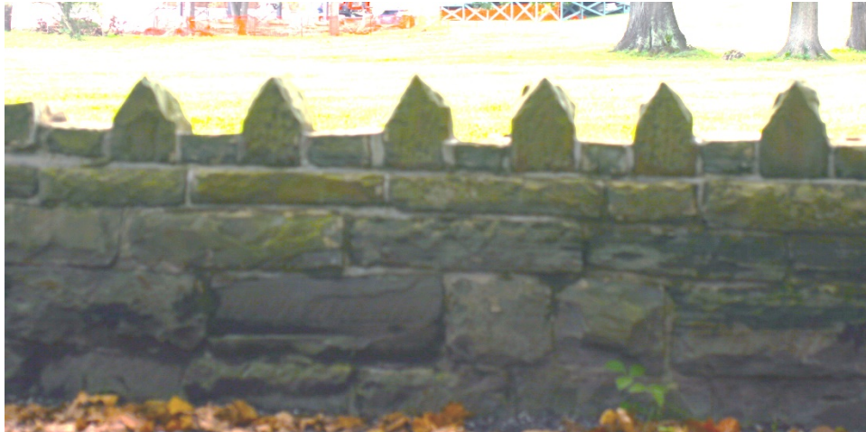
Photo 15 of 19: The c. 1890 knee wall encircling portions of the D & E campus, originally built to enclose “Graceland” and “Halliehurst,” looking west
