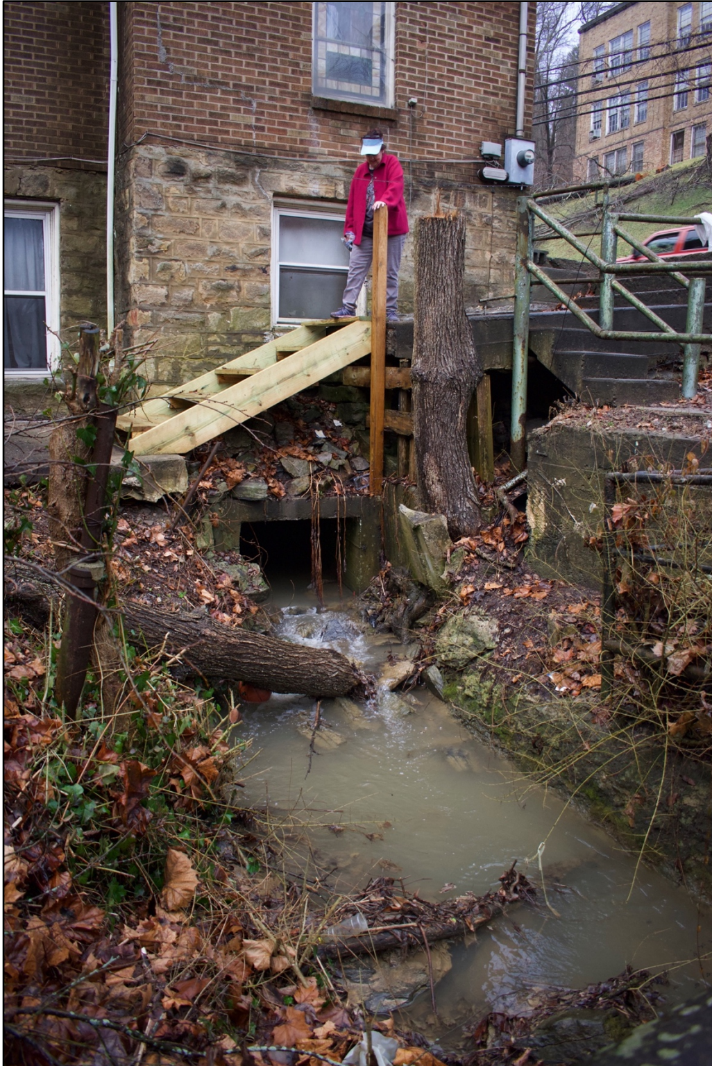
Plate 4. South elevation, facing north. Note 42x36 inch concrete culvert. Photo by Jalon Staples documented January 3, 2023.
