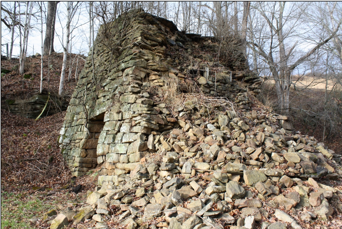
Photo 2. Deteriorated furnace wall, facing north.
