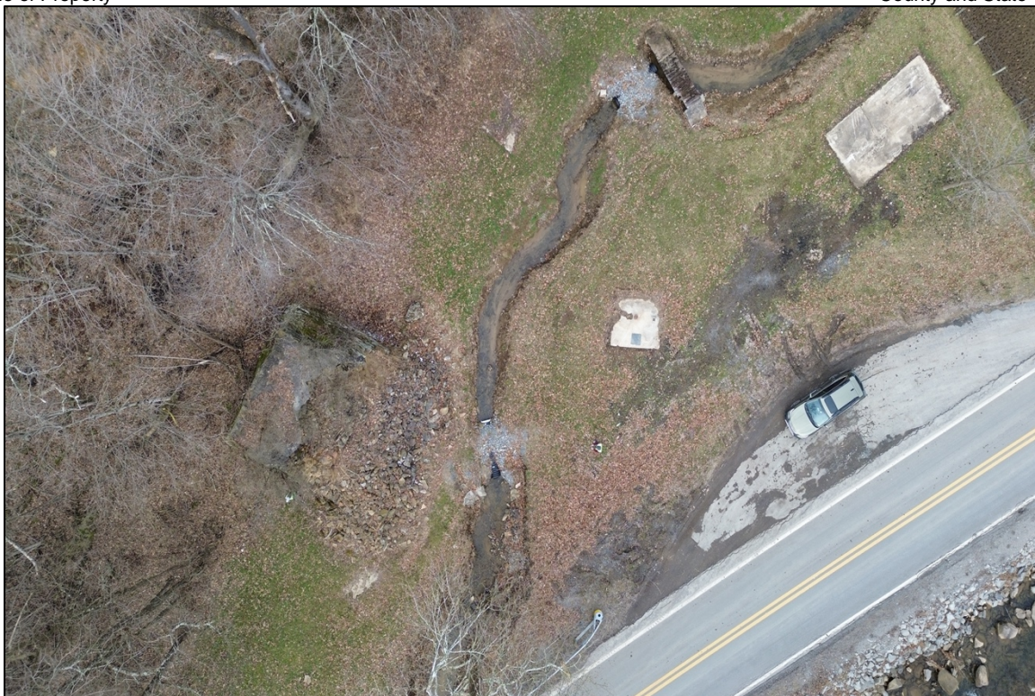
Photo 13. Photograph taken from drone of the furnace site (2/5/2023). Note the deterioration of the southwest side of the furnace.
