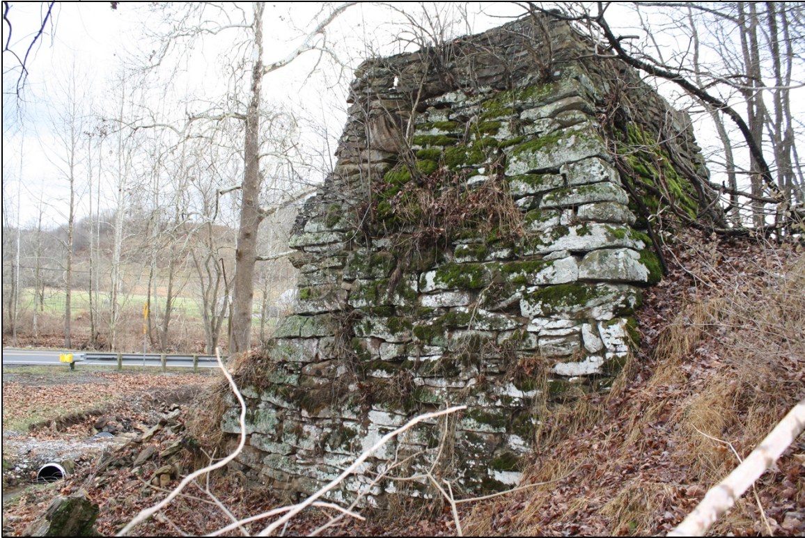
Photo 3. East elevation of furnace, facing southwest. Note hillside banked to the north.
