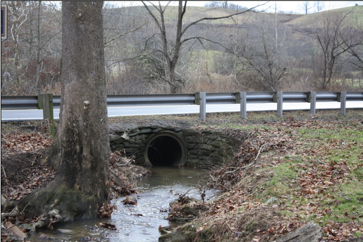
Photo 11. Culvert extending into Brushy Fork. This may have also been a part of the wheel pit.
