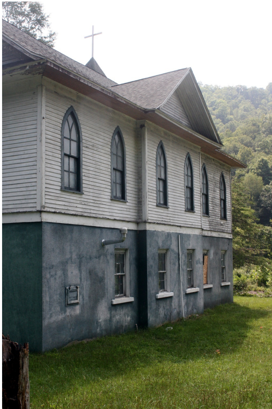
Photo 3 of 10: West side elevation, looking southeast, showing typical side elevation, fenestration, pedimented wall dormer, etc.
