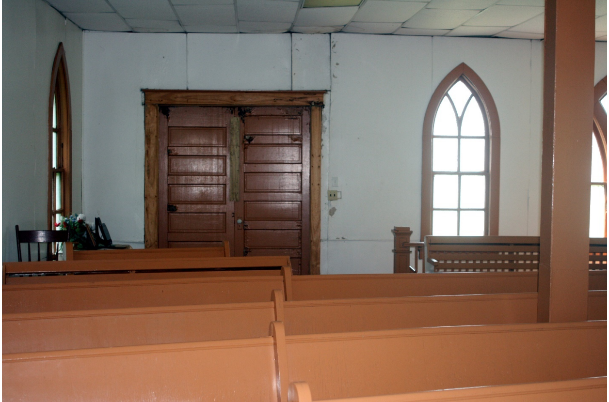
Photo 8 of 10: Sanctuary, view north to south, and showing double-leaf entry doors accessing bell tower and front entrance to church
