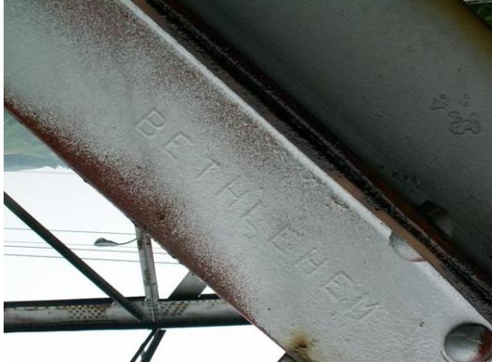
Figure 7: Original steel purchased from Bethlehem Steel Corporation for the Market Street Bridge is stamped with the foundry's name.
