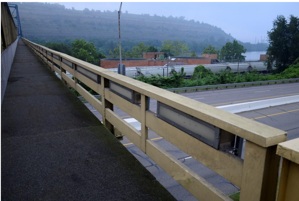
Photo 8: Market Street Bridge, Pedestrian Walk on Downstream side, Note lighting under Handrail Cap, facing East
