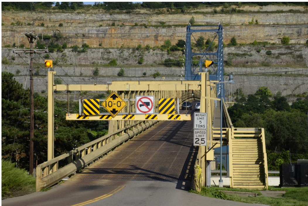
Photo 10: Market Street Bridge, approach on the Ohio (western) side of the river, facing east
