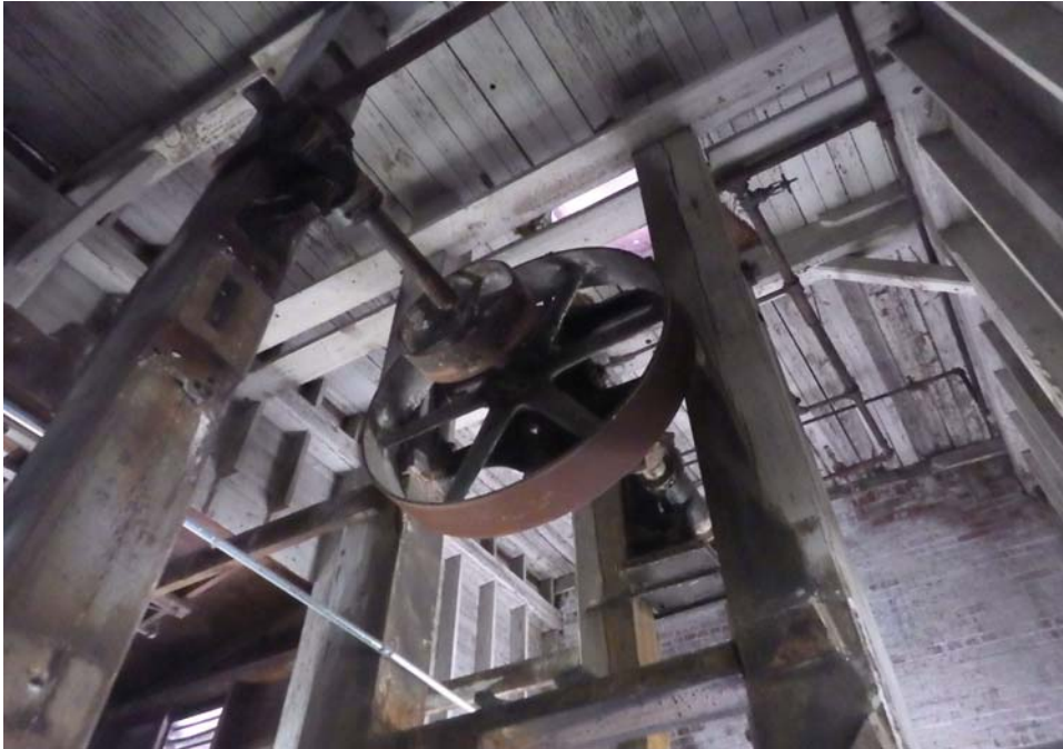
Photo# 15 - Penthouse Fl Original Pulley Wheel
